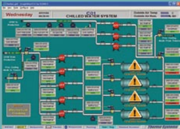
A Thermo Systems Water Chiller Screen
